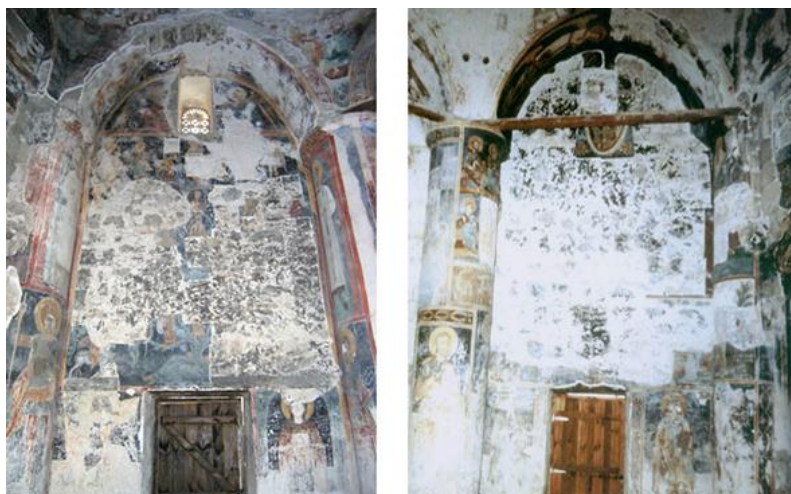
Figure 3 Antiphonitis's church after the vandalism. The north (left) and south (right) walls in the nave with the Last Judgement and the Root of Jesse in the central part.
